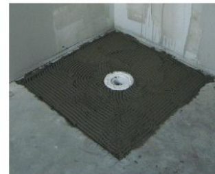
5. Applying tile adhesive onto concrete and special glue onto PVC leak control flange
